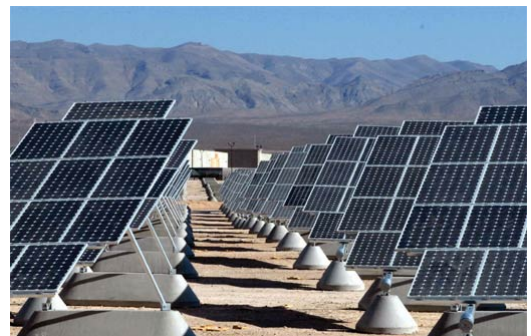
Sarnia Photovoltaic Power Plant (カナダ)
